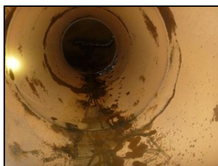
Figure 1 Abrasion-corrosion in suction pipes of dredgers. Picture courtesy: Jan De Nul
